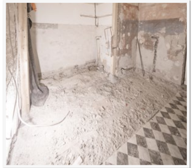
From practical experience: uneven floor after tile removal.
